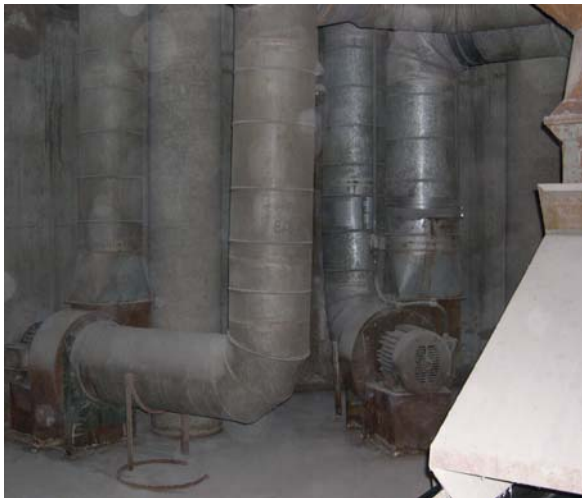
Current situation with fans located inside structure.
